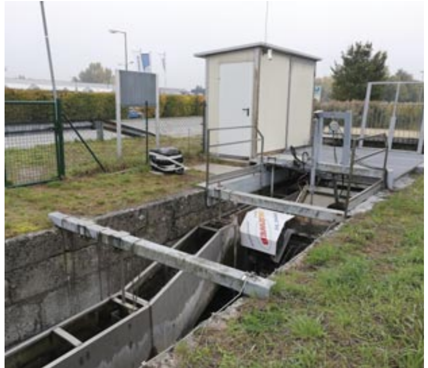
Hydroelectric power station at the Wiener Neustadt Canal, sluice 2, Gumpoldskirchen
