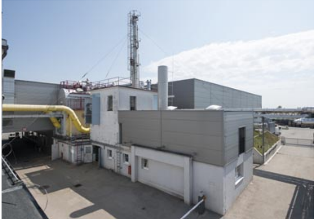
View of the solvent recovery plant
