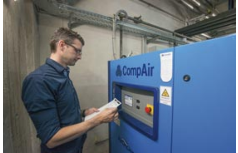
René Blumauer in front of the new compressor
