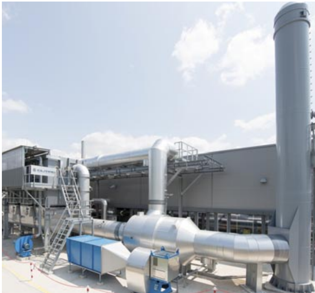
This is what air quality control looks like - the new RTO for exhaust air purification
